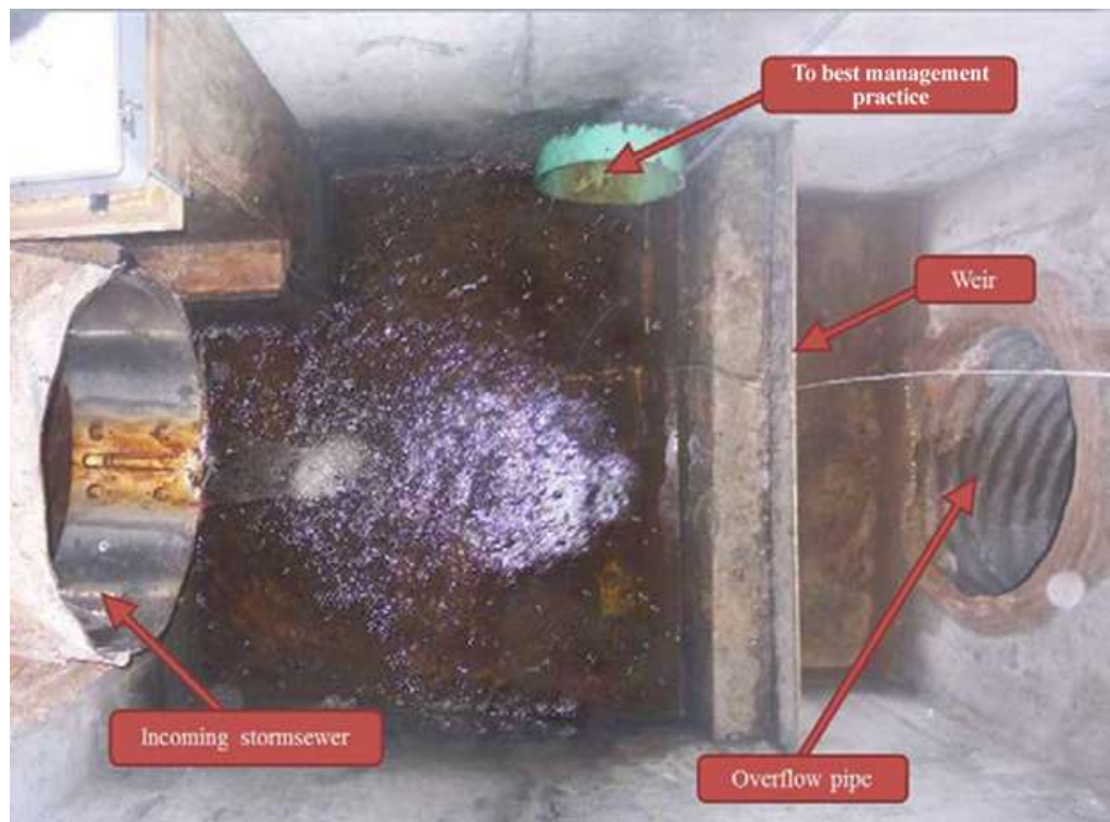
Figure 10.8-3 - A commonly used flow bypass structure configuration that bypasses flow when the capacity of the outlet pipe supplying the BMP is exceeded (photo courtesy of NCSU-BAE)
