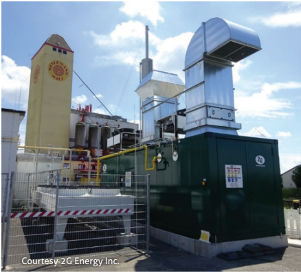
The Hassfurt green hydrogen CHP system – the first municipal application of the technology.
