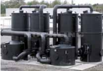
Polystone® G black B 100 Air purification system in a water treatment plant
