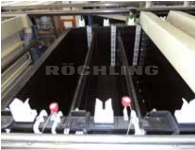
Tanks made from Polystone G HD black in an electroplating plant
