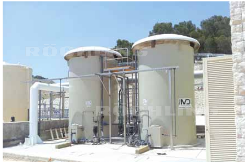
Bio filters for odor neutralisation
