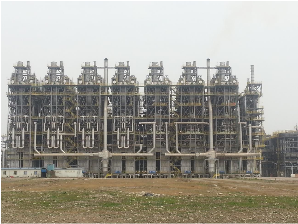
Figure 2: The above picture shows the eight cracking furnaces operating with the Zeeco GLSF Enhanced Jet flat flame burners, which produce measured NO x emissions between 35 mg/Nm 3 (17 ppmv) to 65 mg/Nm 3 (32 ppmv) at design heat release. From the picture, one can see seven furnaces are twin cell furnaces and one furnace is a single cell furnace.
