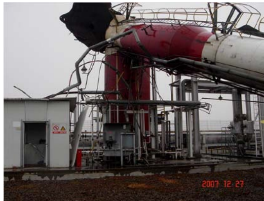
Figure 15. Destroyed Flare Stack as Result of Flashback
