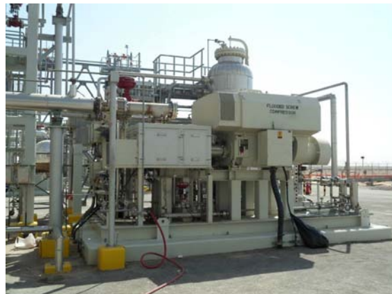
Figure 13. Zeeco Flooded Screw Compressor Skid
