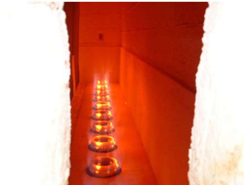
Freejet™ Burners in Dow Chemical Ethylene Cracking Furnace Freeport, Texas
