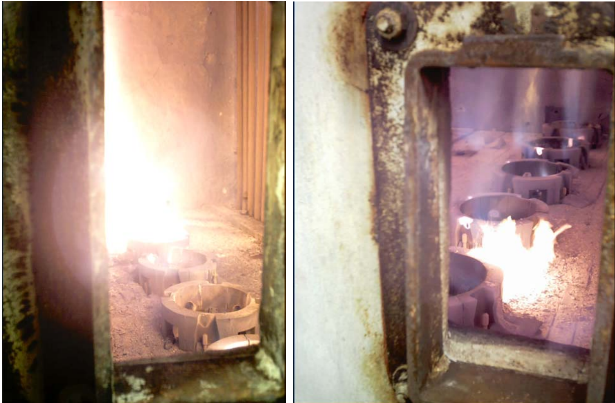
These pictures depict poor flame quality.
