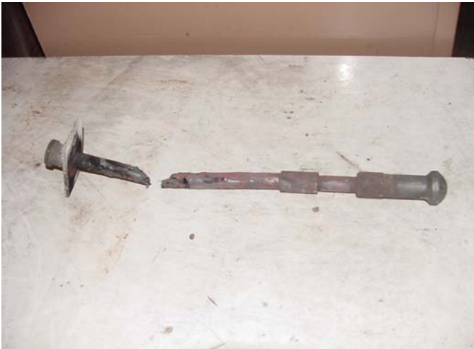
Typical exposed Gas Riser failure
