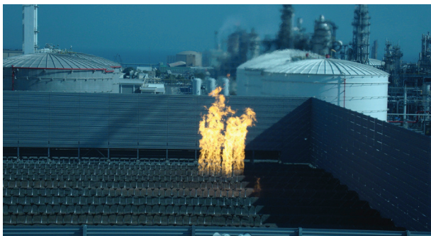
Figure 1. Typical multi-point ground flare installation.
