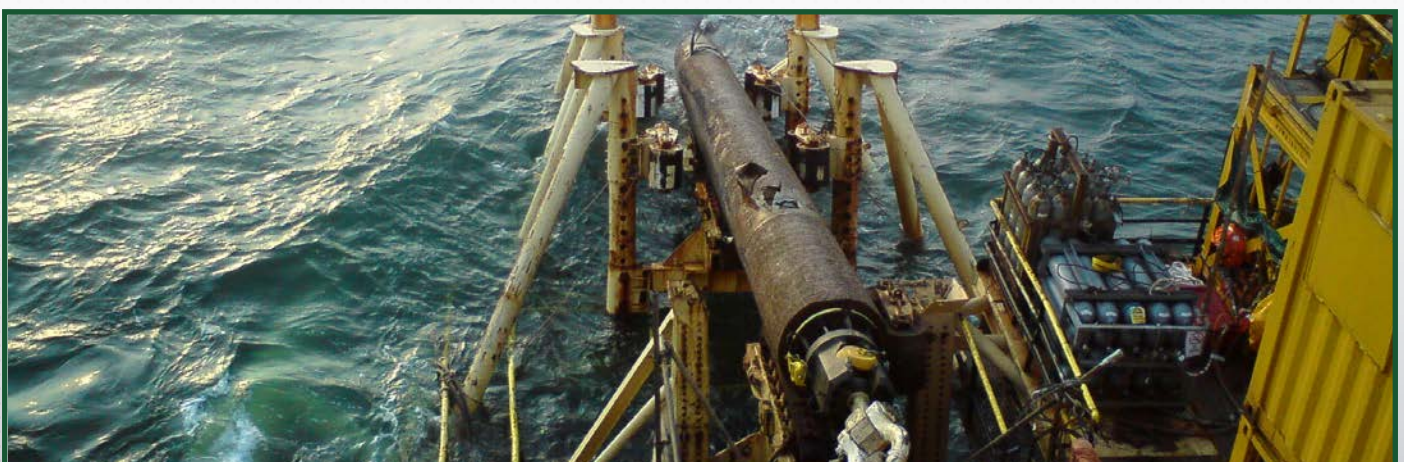
Pipeline Retrieval Tool Recovers Damaged Pipeline to the Surface
