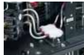
Coated Electrical Connections
