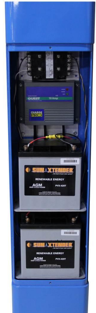
PCS-84-10 shown with PCS-SD-277-350 and housed in ETP-MTE Tower Mount
