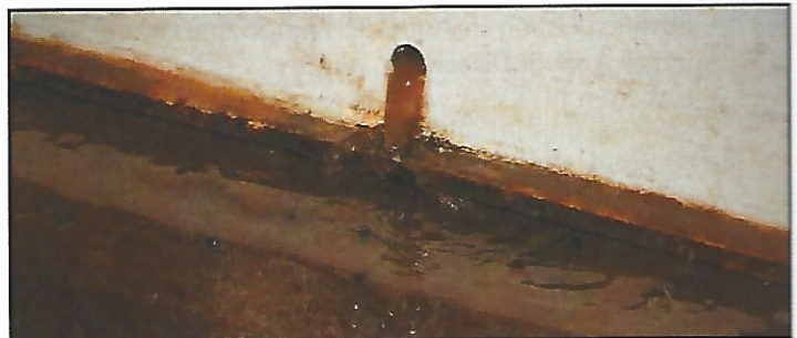
Figure 2 Adsorption Clarifier buoyant media had been leaking from the unit's weep hole.
