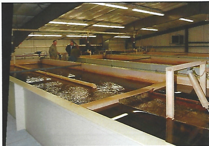
Figure 1 Twenty-one years in operation had taken a toll on the original system.
