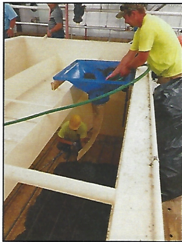
Figure 3 Filter bed media was installed atop the new in-bed air grid for air-water backwashing
