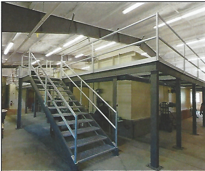
Figure 6 Three tank treatment units
