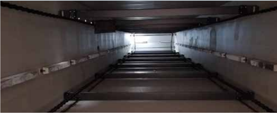
The oil water separators are constructed of corrosion-resistant materials inside and out.
