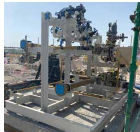
The three pump skids remove sludge from the separators' sludge hoppers.
