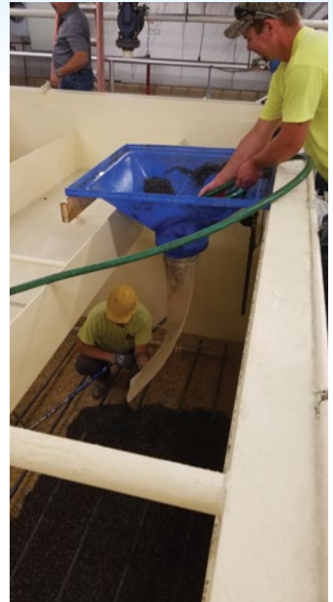
Filter bed media was installed atop the new in-bed air grid for air-water backwashing.
