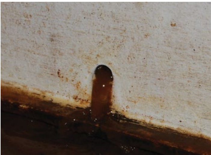
Adsorption Clarifier buoyant media had been leaking from the unit's weep hole.
