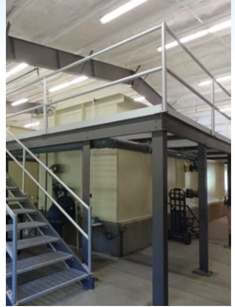
Simple but necessary upgrades to the Trident system improved plant efficiency.
