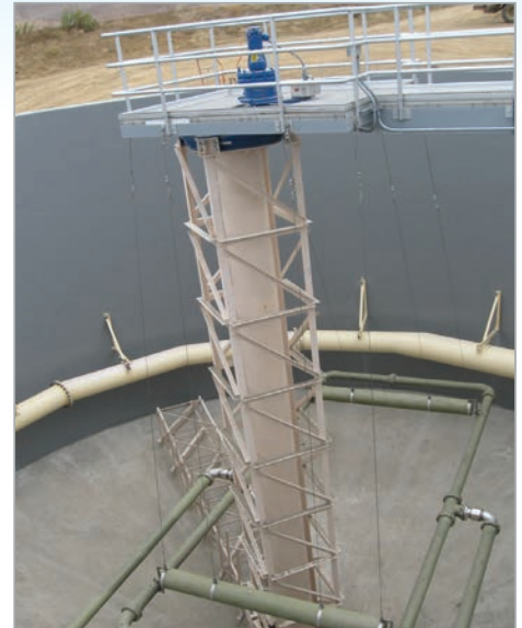
Fill and Decant Clarifier
