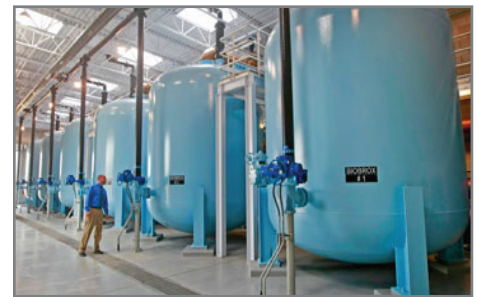
Magna Water Treatment Plant in Operation
