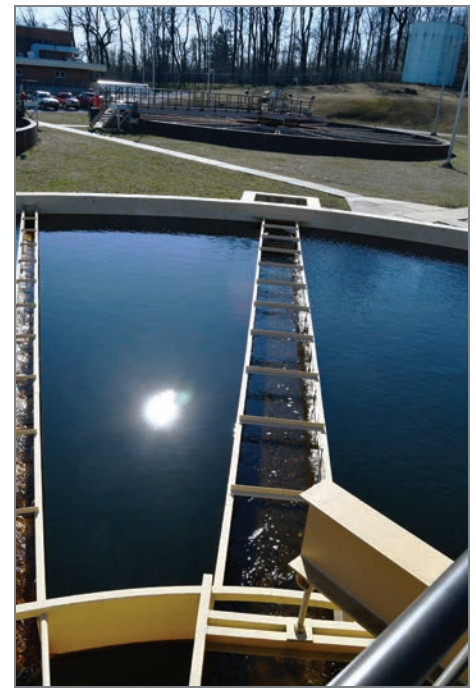
New and retrofit CONTRAFLO units on-site at the City of Lebanon Authority WTP
