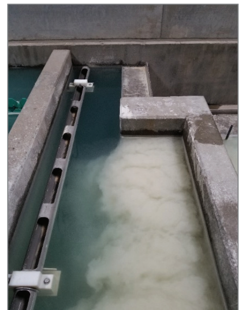
Picture of solids in properly operating clarifier
