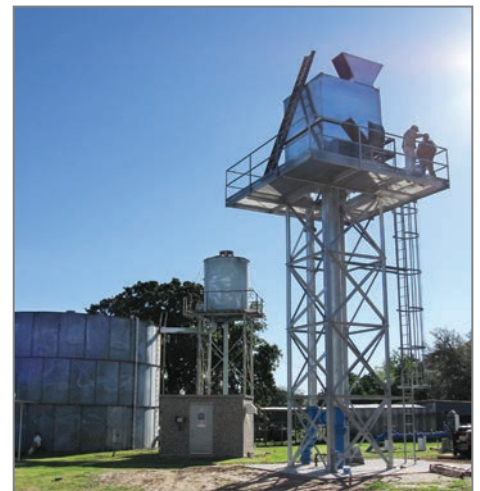
Existing and New Forced Draft Aerators
