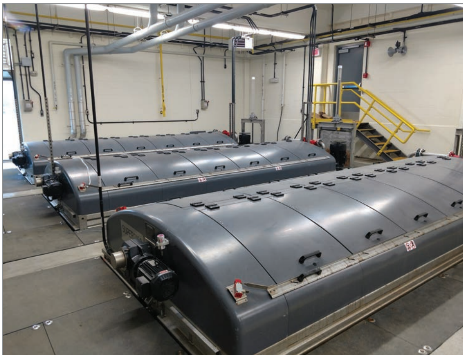
The plant's three-unit SuperDisc phosphorous removal system
