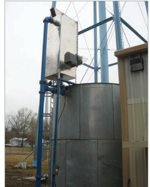
Forced Draft Aerator
