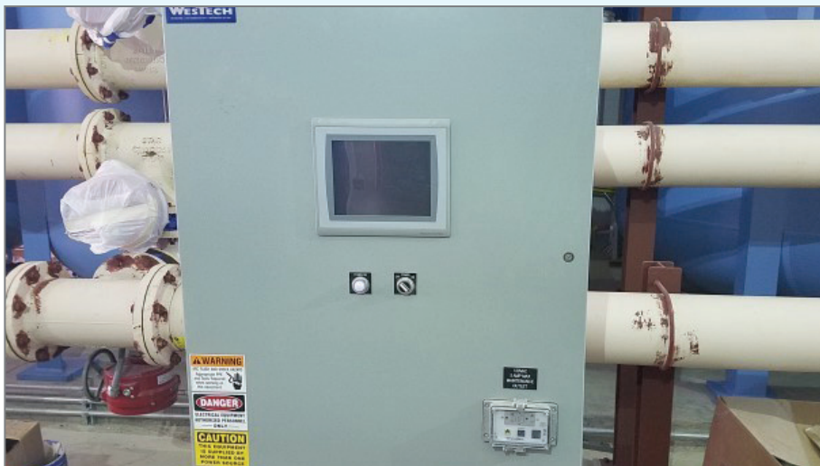
BWSD's PLC-SCADA system
