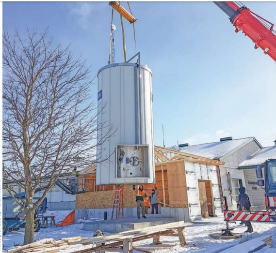
A double-pulley crane lifted the tower horizontally from the truck then turned it upright to place on a 12-by-12-foot concrete pad next to the milk house addition at Grootendorst Farms.
