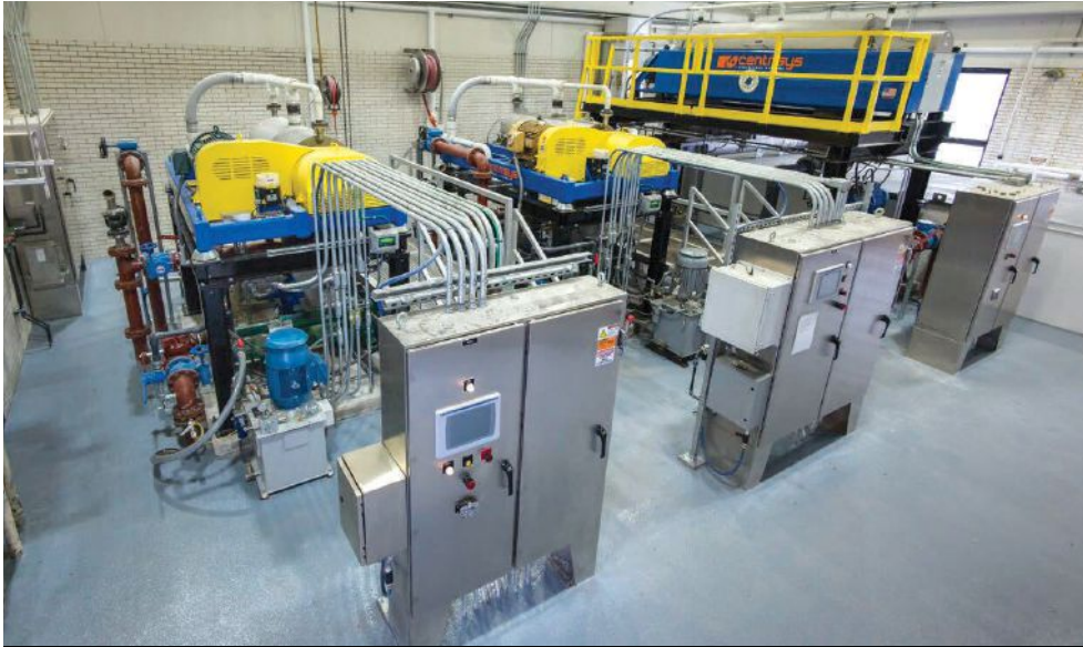
Image 2. The centrifuge room at the Kenosha Wastewater Treatment Plant. Pictured are the plant's three centrifuges including a pair of thickeners for primary sludge and waste-activated sludge, and a dewatering centrifuge.
