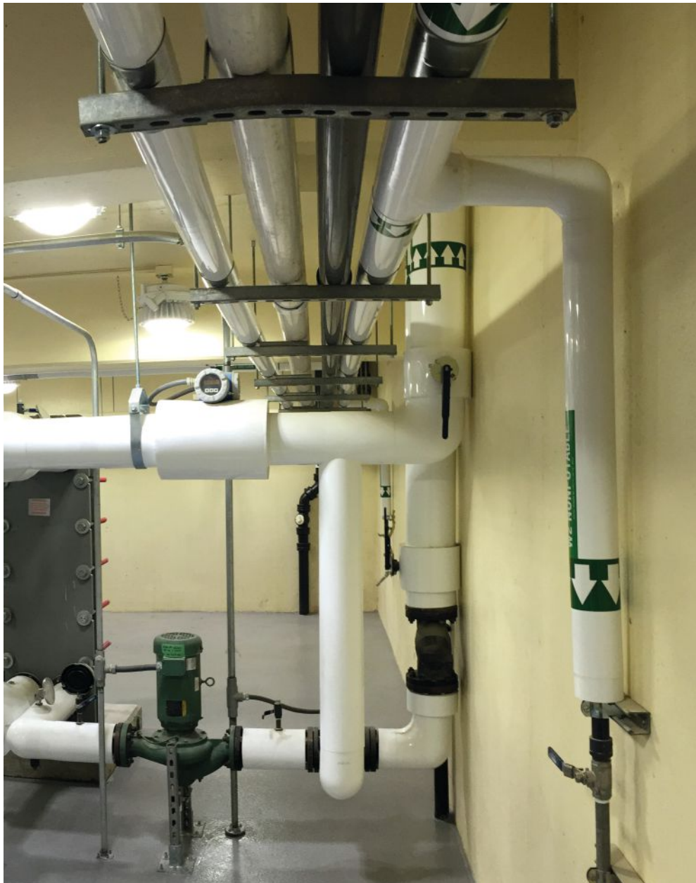
Image 1. Pumps and heat exchanger linked to the reactor as part of the process to capture and transfer methane for reuse as biogas. (Images courtesy of CNP Technology Water and Biosolids Corporation)
