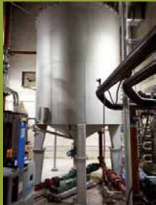
The Kenosha Wastewater Treatment Plant's PONDUS process hydrolyzes waste-activated sludge.
