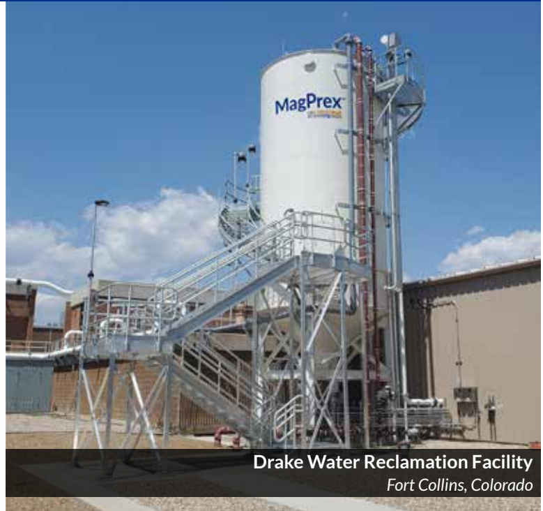
Metro Water Recovery Denver, Colorado
