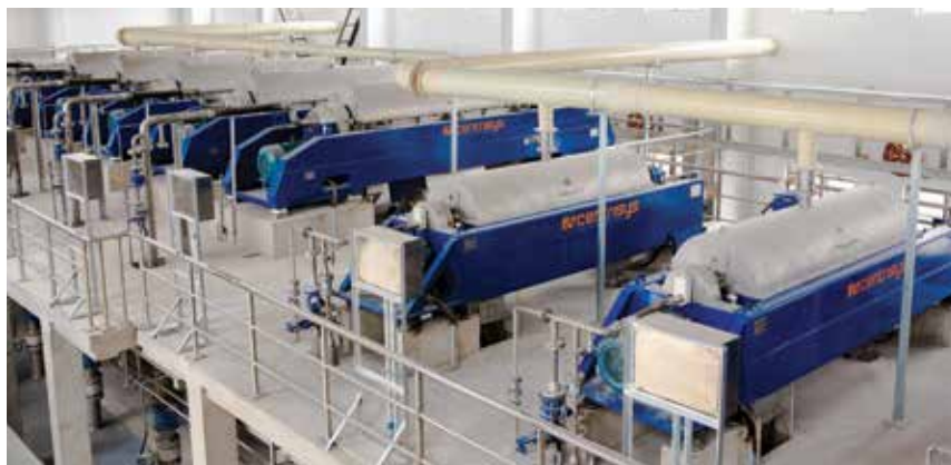
DingFuZhuang WWTP Beijing, China: Five Centrisys THK600 and four CS21-4HC.
