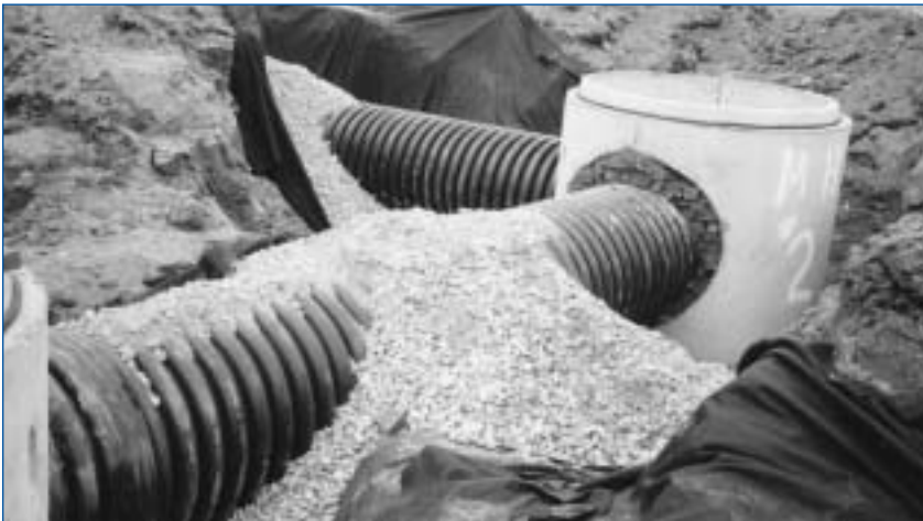
36-inch HDPE drainage header
