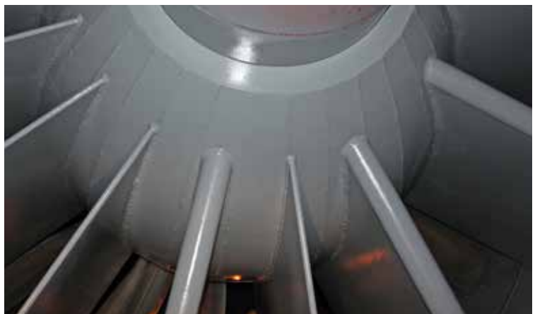
The fan blades now coated with ChemLine® in this close-up inspection photo shows excellent performance against the corrosive flue gas/chemical service conditions.
