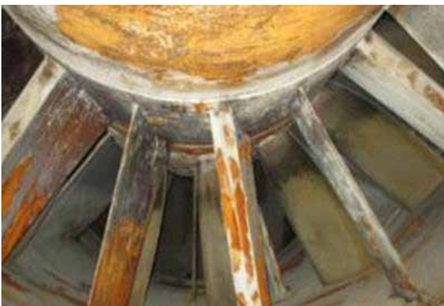
(Left) At this coal-fired plant, the carbon steel booster fans in the FGD stacks exhibit severe corrosion problems and need to be coated. (Right)
