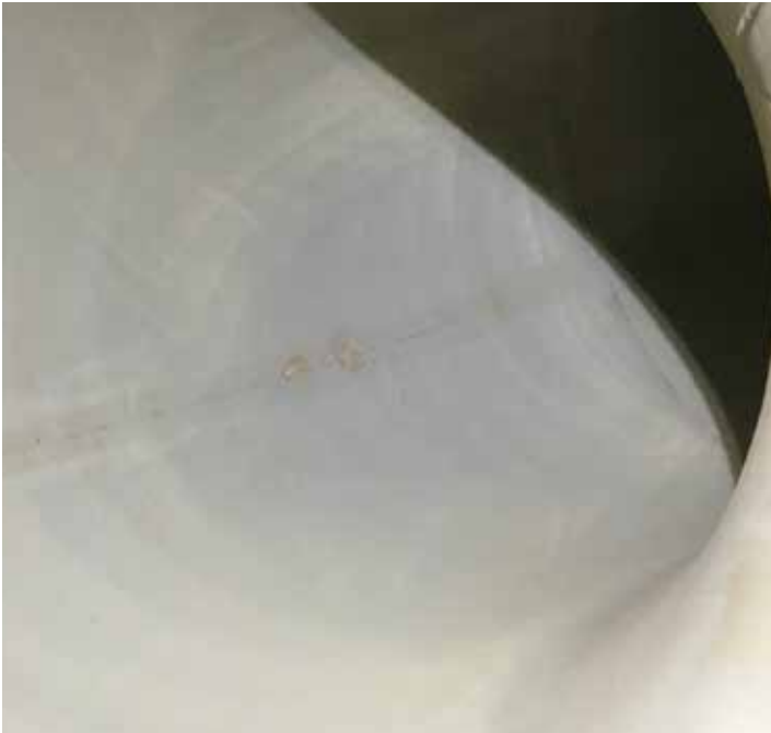
CONDENSER LINE AFTER 1 YEAR CHEMLINE® SERVICE
