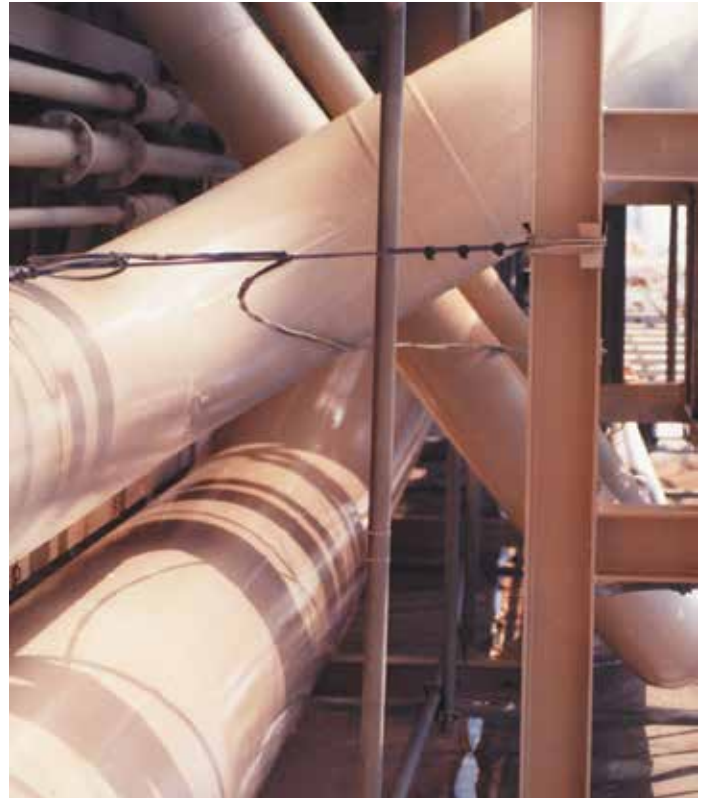
Pipe running throughout Tonen facility is coated with ChemLine®.
