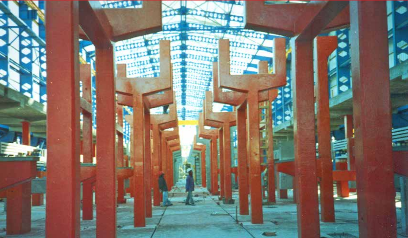
Concrete electrolysis tank support pillars are coated with ChemLine®.
