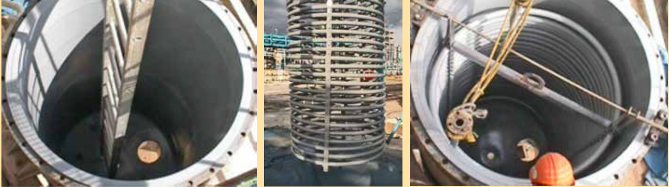
(Left) Re-lining the R-310 reactor vessel with ChemLine®. (Center) ChemLine® coating of the stainless steel coil used in the reactor. (Right) Reactor and coil, both coated with ChemLine®, ready for service again.
