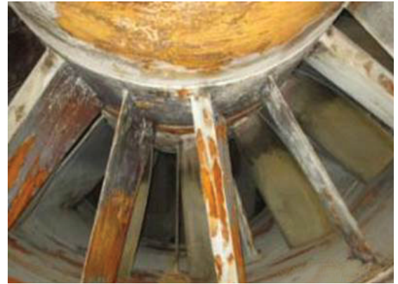
Booster fans exhibit severe corrosion problems and need to be coated.
