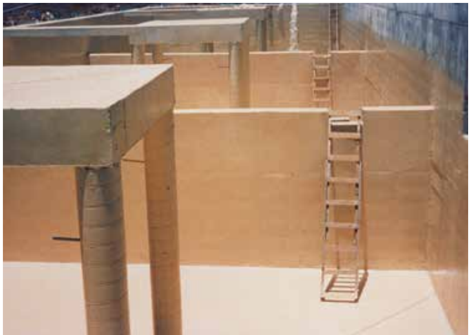
Secondary containment areas at B.F. Goodrich holds various chemicals.
