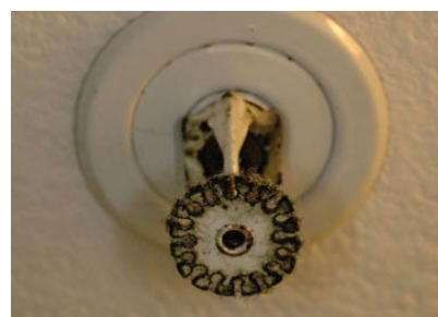
Corroded Sprinkler Head
