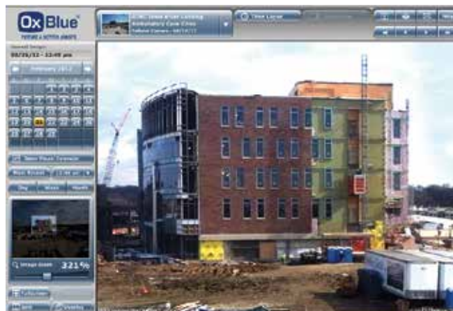
A view of the UIHC Iowa River Landing Ambulatory Care Clinic from an OxBlue construction camera.
