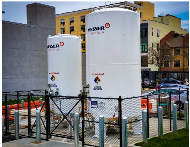
In the midst of uncertainty around COVID-19, Virtair and Messer went above and beyond to execute a safe and timely bulk medical oxygen installation at Brooklyn Center for Rehabilitation and Residential Healthcare.
