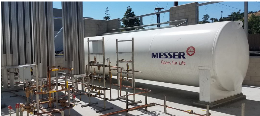
The main and reserve vaporizers and main O 2 tank after installation at the LLUMC bulk O 2 compound. The bracing is in the base plate, the saddle and the anchors into the outer shell of the tank.
