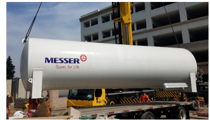
Messer lowers bulk O 2 tank into place. The new bulk O 2 compound is across the street from the new hospital, then under construction, at LLUMC.
