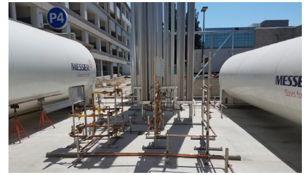
The main (left) and reserve tanks, plus the vaporizers and associated piping at the LLUMC bulk O 2 compound.
